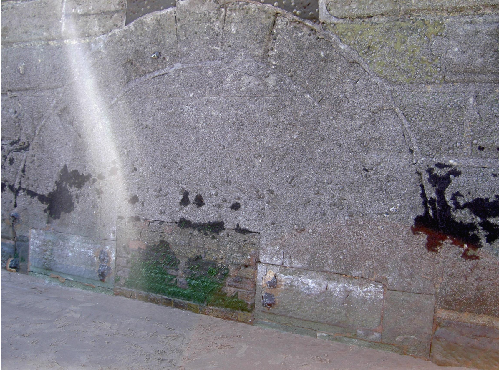
Margate Harbour Sluice –Portland Stone and Brick sealing wall to culvert viewed from outer face of Stone Pier
